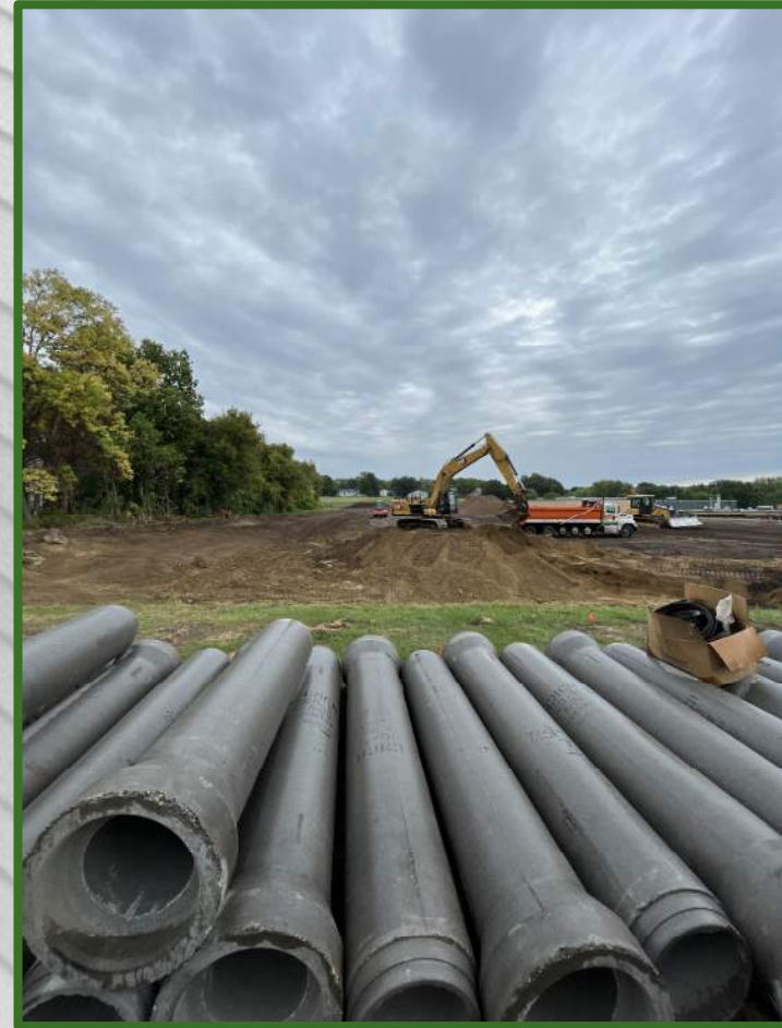
Final excavation and exporting of soils from retention pond (sewer pipe is for ES bus loop)
