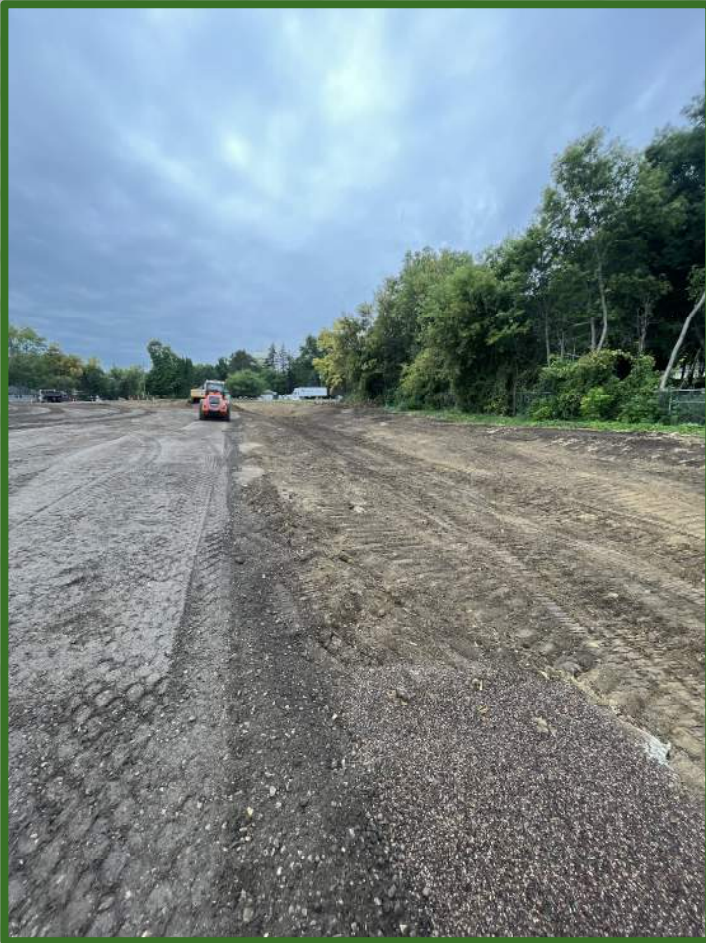
Storm sewer piping and structures installed along Western edge of bus loop
