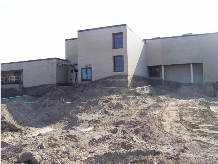
09/15/15 This image shows the amount of excavation at the building pad for the new west addition.
