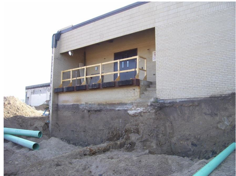
09/15/15 This image shows the depth of subcut at the existing loading dock.
