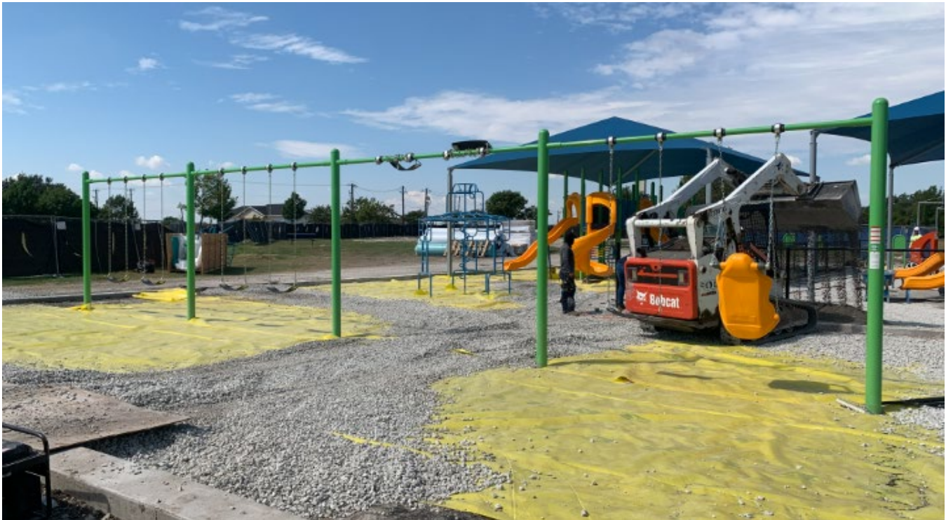
The surface of the new playgrounds (Abbett pictured above) is designed to drain quickly and last many years.
