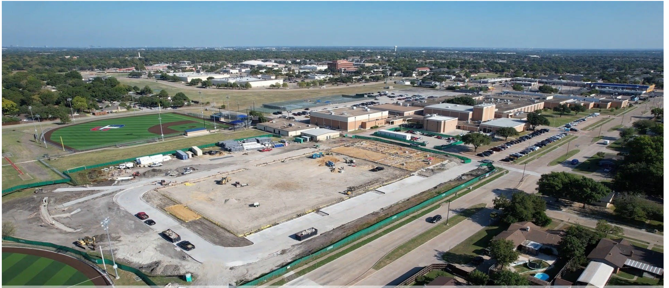
South Garland High School
