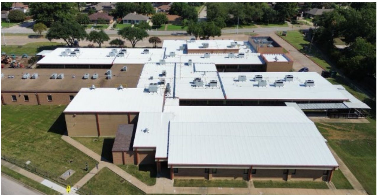
The new 2-ply modified bitumen roof at Cooper ES will last for many years.
