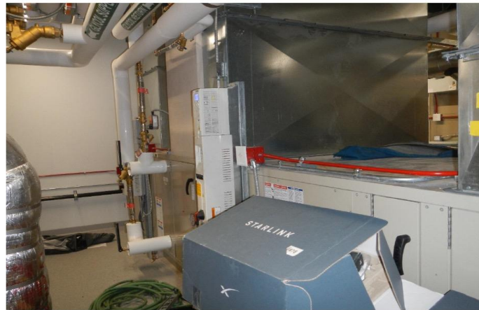
Figure 35 Clutter needs to be removed from all mechanical rooms
