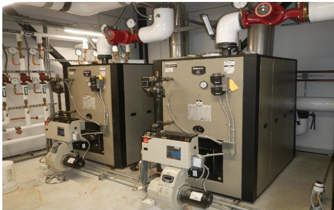
Figure 39 One of the boilers has not worked since the opening of the school 2 years ago
