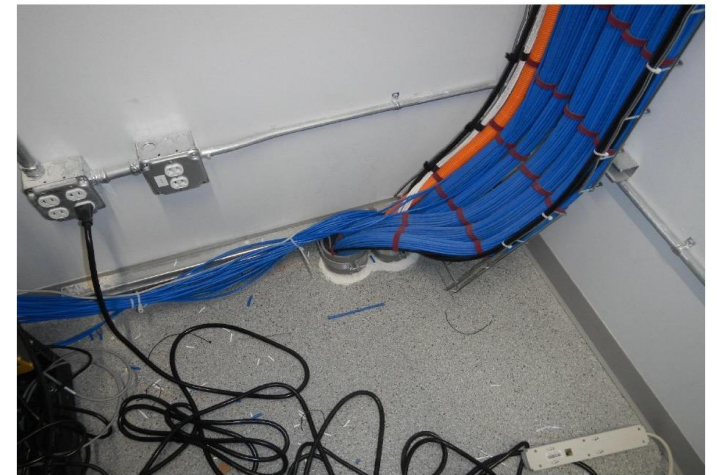
Figure 37 Trip hazards in network room
