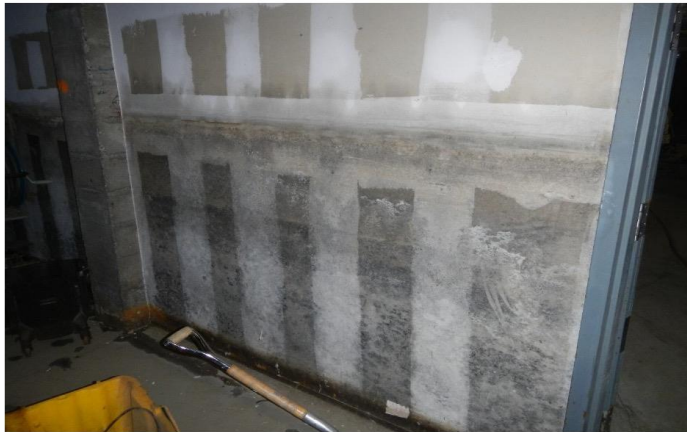
Figure 27 Water damage from typhoon flooding
