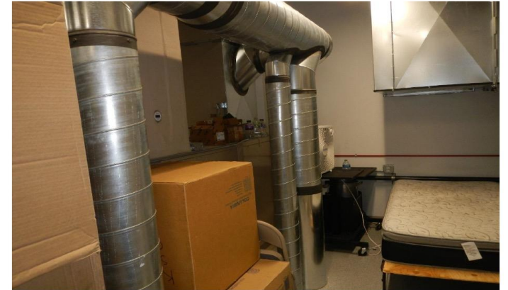
Figure 36 Clutter must be removed
