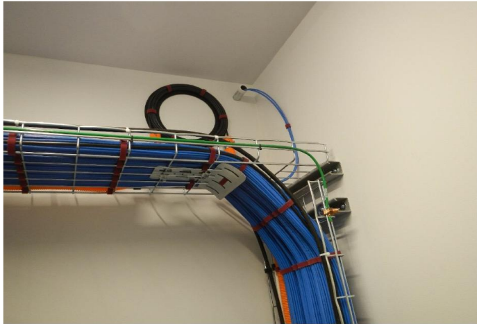
Figure 38 Firewall penetrations must be sealed
