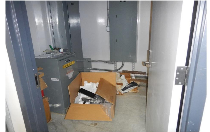
Figure 42 Nothing can be blocking the electrical panels. Electrical rooms must be clutter free
