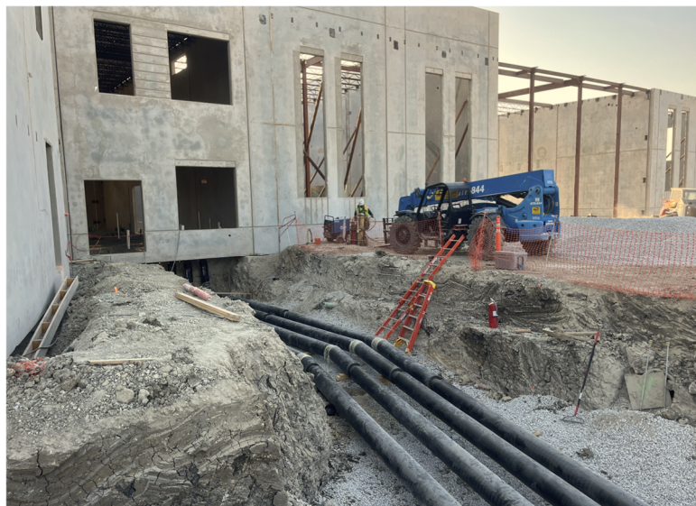
Hydronic Piping Entering the Building
