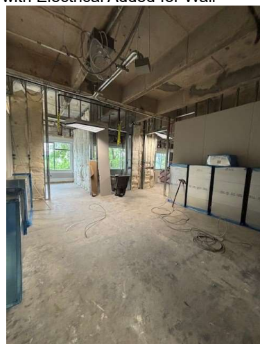
2nd Floor – Esthetician Reception Area with Intake Offices, Insulation and One-sided Walls
