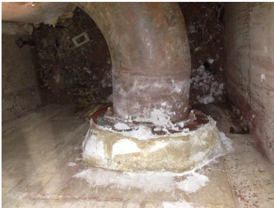
Picture 4 (Temporary patch Fall 2014)
