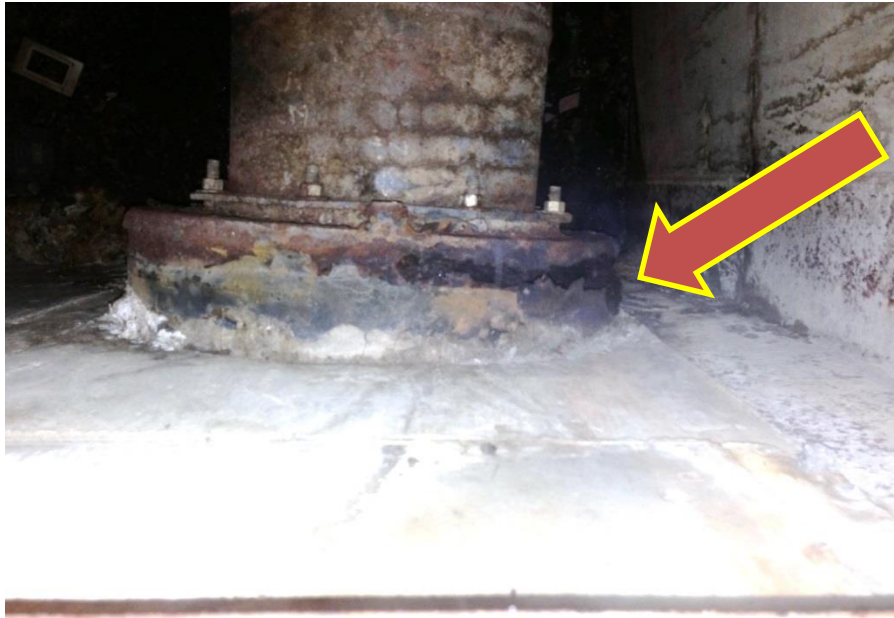
Picture 3 (Steam pipe insulated jacket starting deteriorate)
