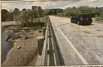
A vehicle passes over the bridge spanning the West Fork of the White River on Thursday along Main Street in West Fork. The city of West Fork is working with the Arkansas Department of Transportation to replace the bridge with work set to begin in 2025. Visit www.democrat-gazette.com for today's photo gallery. (NWA Democrat-Gazette/Andy Strupe)
