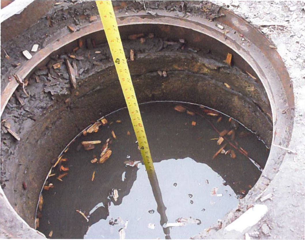
Clogged upstream structure (above)
