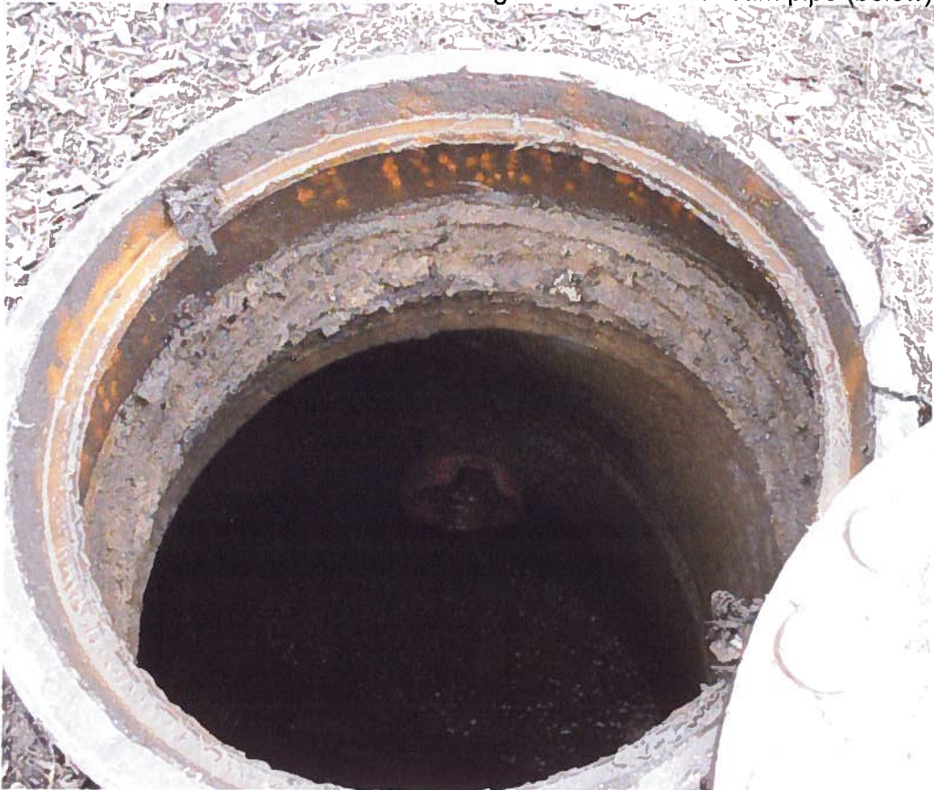
Water trickling out of the downstream pipe (below)
