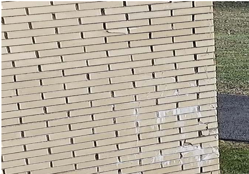
Tuck pointing needed.
