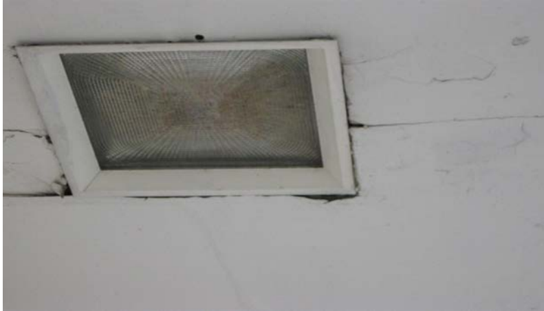
Replace exterior lighting.
