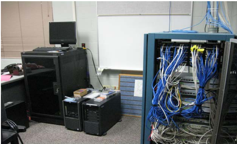
Crowded server room/equipment.
