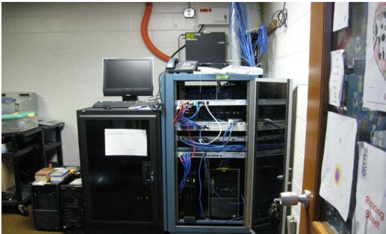
Crowded server room/equipment.
