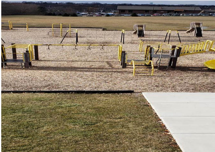
Aging playground equipment.
