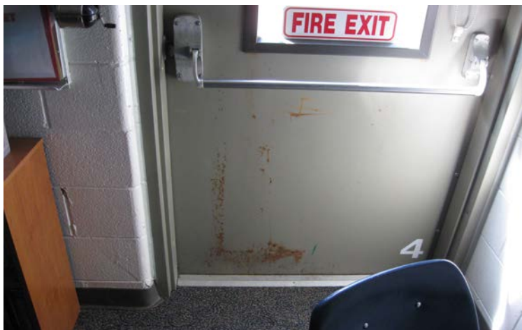
Exterior door needs replacing.
