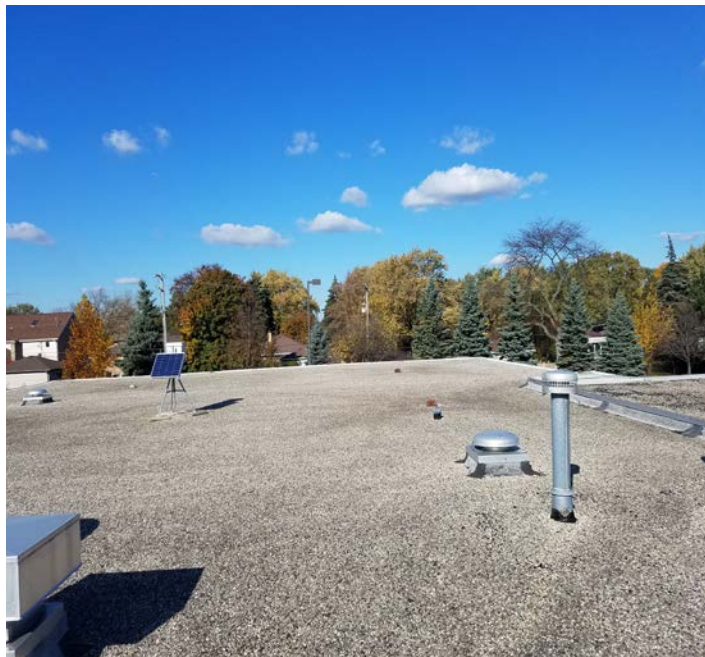
Roof is aging.
