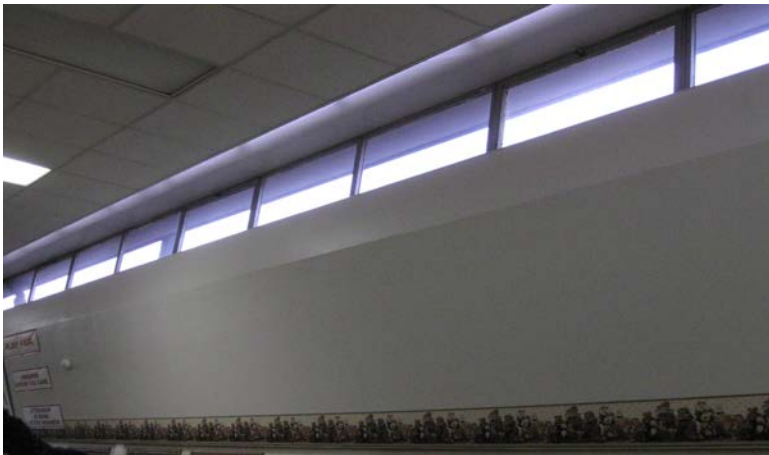
IMC windows need replacing.
