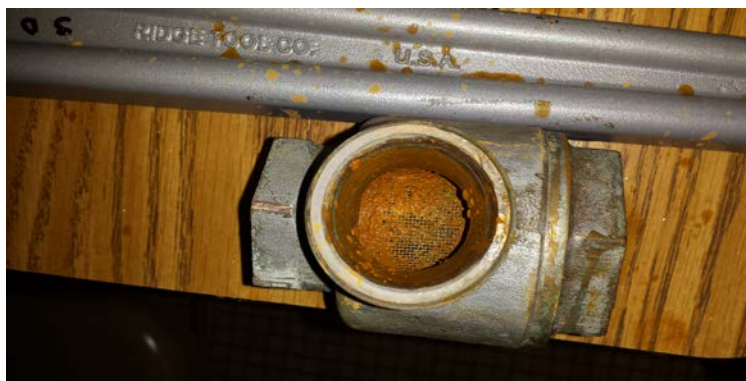
Rusty pipe fitting.
