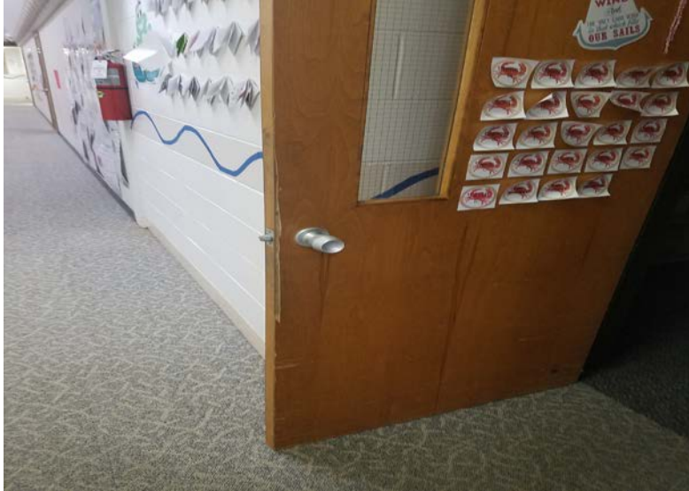
Classroom doors needing replacing.
