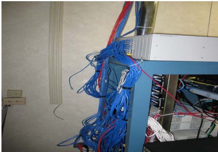
Server room switch gear and cables.
