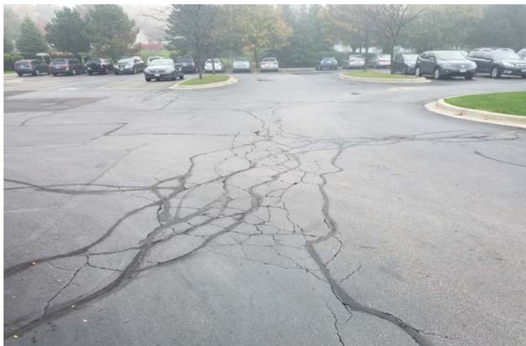
Parking lot patching needed.
