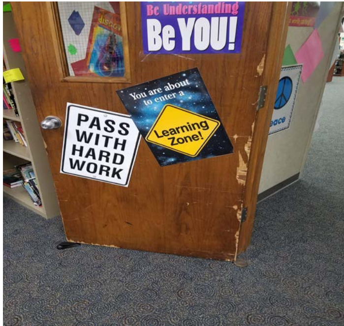
Interior door needs replacing and doorknob not meeting ADA requirements.
