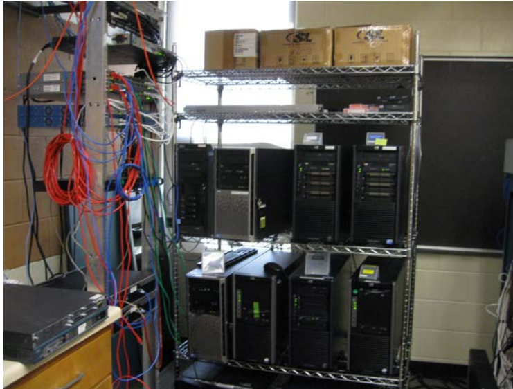
Server room equipment.
