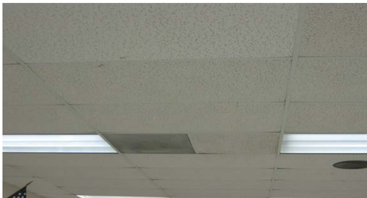
Sagging, old ceiling tiles.
