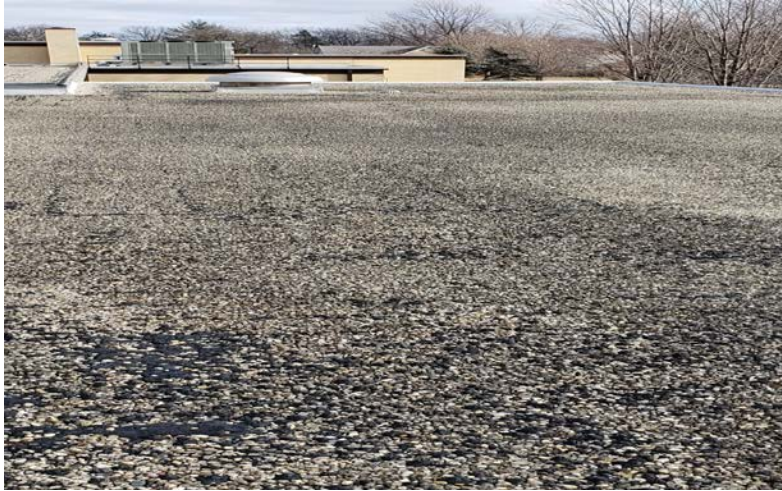
Roof needs replacing
