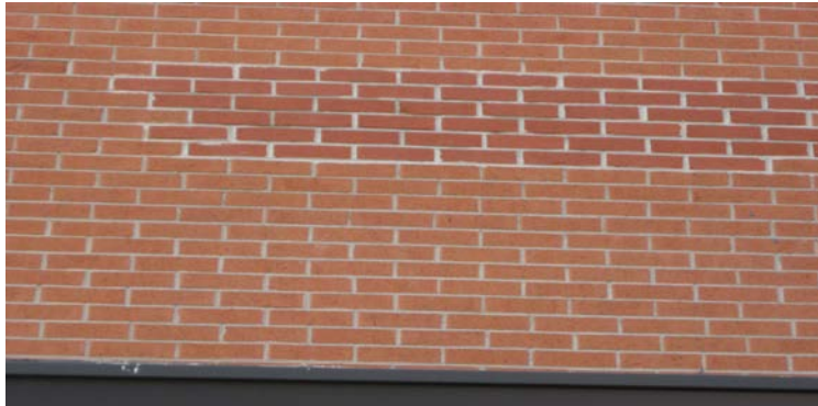
Replacement brick difficult to match.
