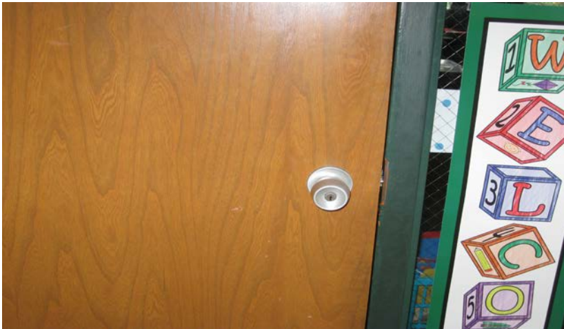
Door hardware not to ADA guidelines.
