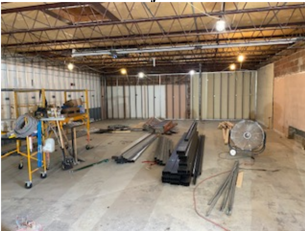
Figure 1 The pits in the two music classroom floors have been filled in with sand and concrete.
