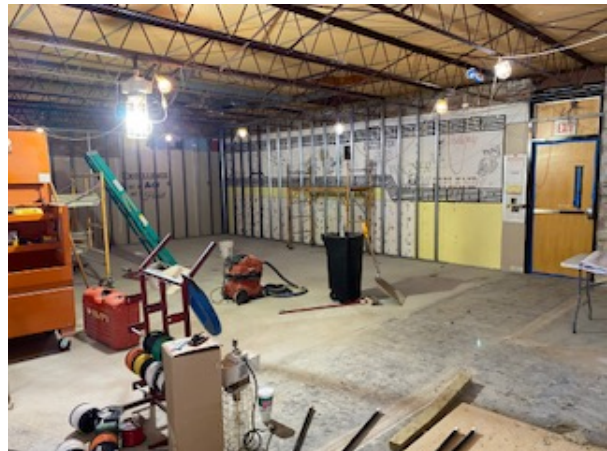
Figure 2 Steel studs are going up against the walls so that drywall can be mounted to smooth the walls.
