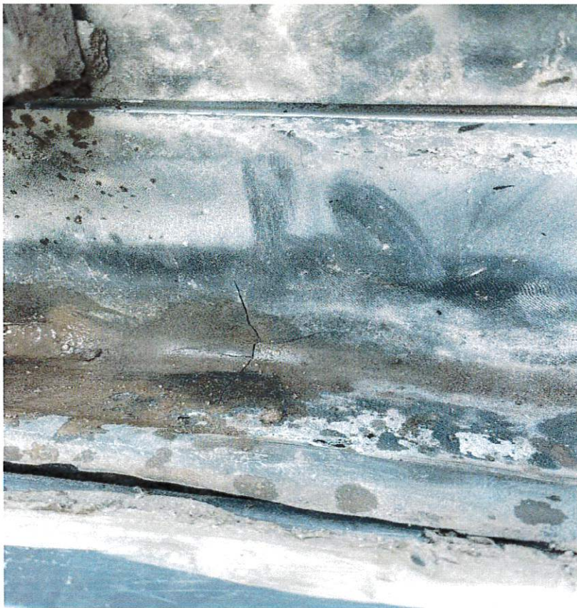
Though wall flashing is cracked at horizontal/vertical transition @ test cut area.
