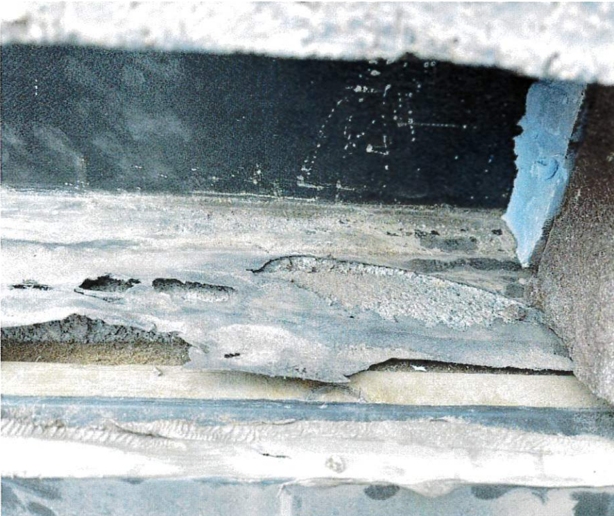
Through wall flashing appears to be worn through in multiple location @ test cut area.
