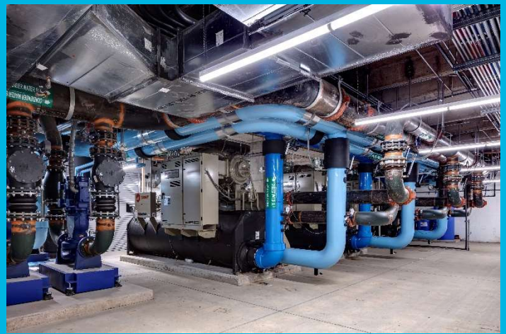
Central Utility Plant Chiller and Pump Room
