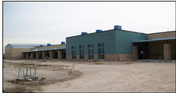
New Elementary School: $97.00 s.f.
