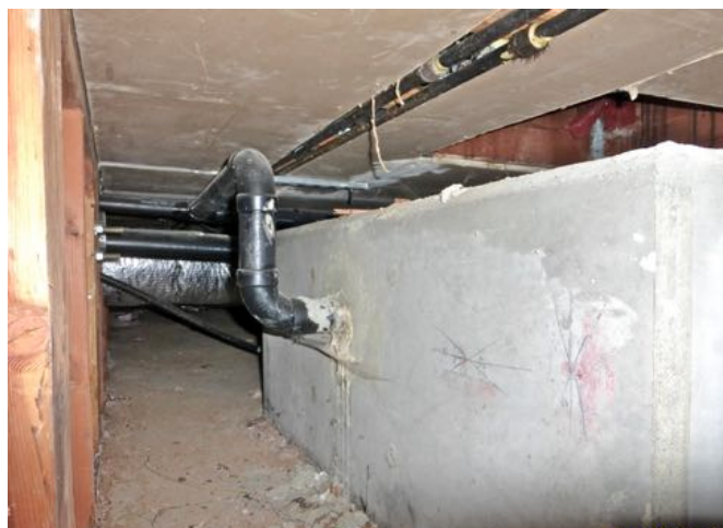
Crawl space and treatment tank
