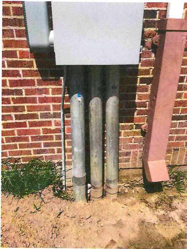
Missing straps and Unistrut for disconnect serving building "C".
