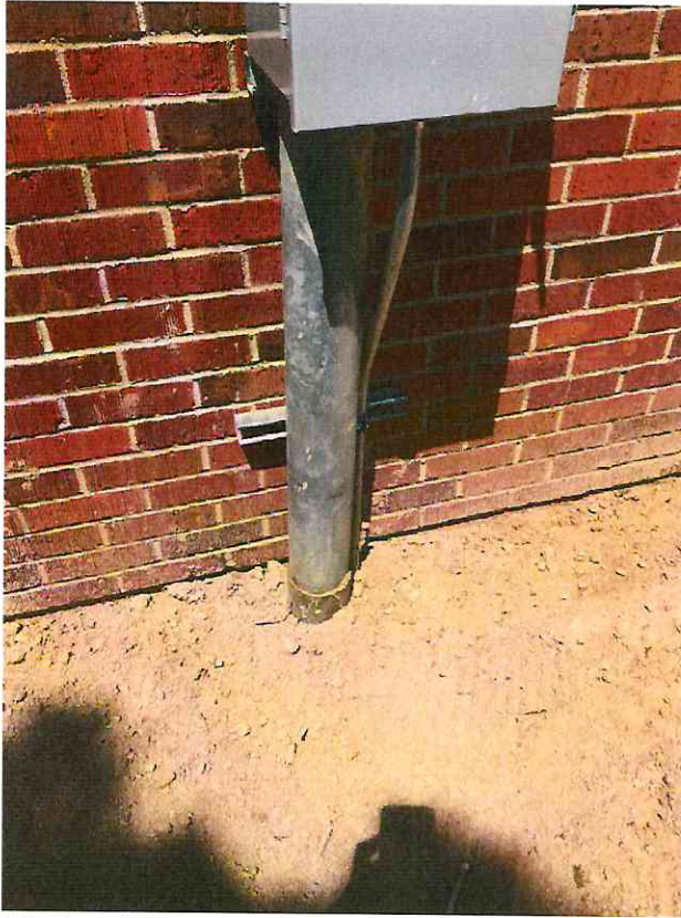
Missing strap at Unistrut for disconnect serving building "A".
