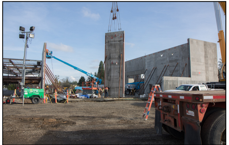
Precast panel in gym
