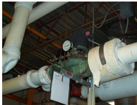
Primary Boiler Pump
