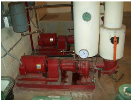
Secondary Boiler Pump
