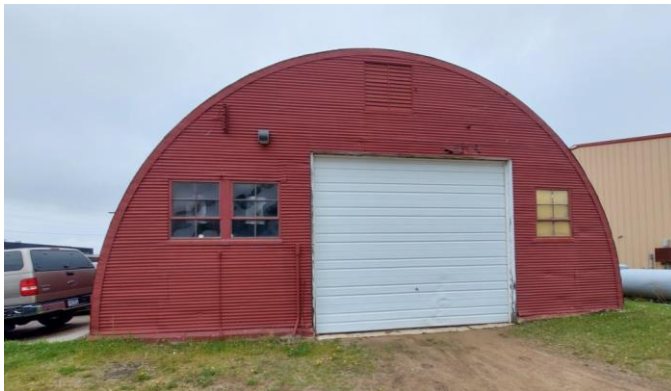
11: Large, manual opening garage door
