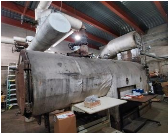
4: Steam boiler past its useful life
