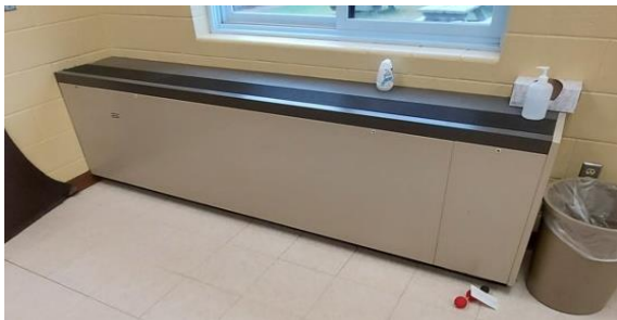
5: Unit ventilators are past their useful life
