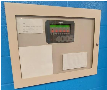
8: Problematic fire alarm control panel
