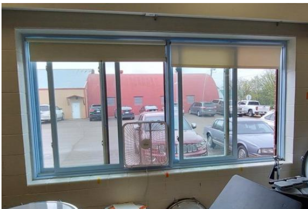
6: Sliding windows are open often to help ventilate rooms
