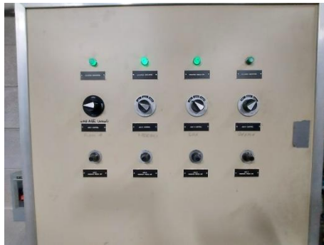
7: Outdated pneumatic controls
