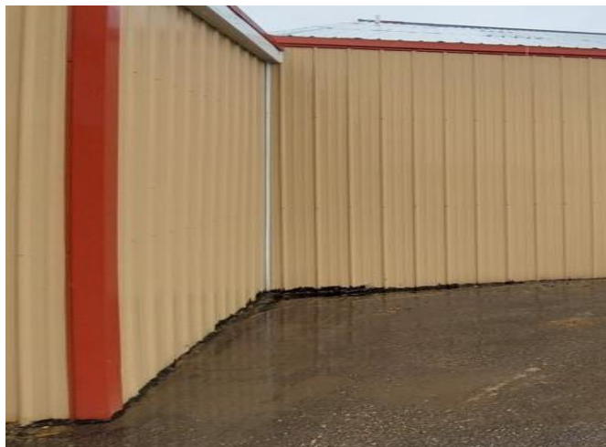
12: Pavement slopes towards the building causing water infiltration
