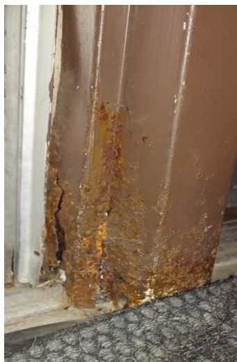
9: Heavily damaged door frames that are rusted through
