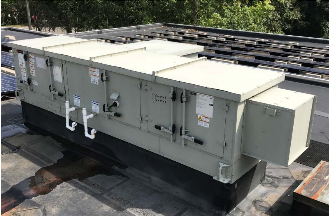
Figure 9- Typical Rooftop Unit (not in scope of evaluations)
