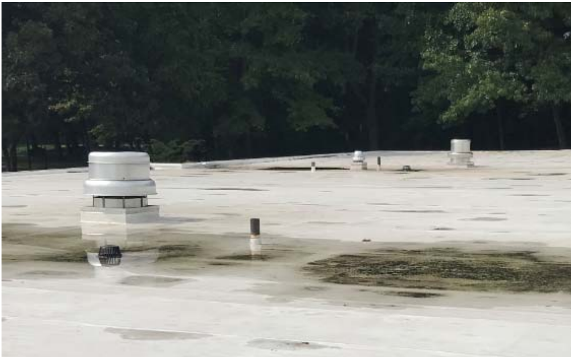
Figure 6- Typical Roof Mounted Exhaust fans serving classrooms with UV's
