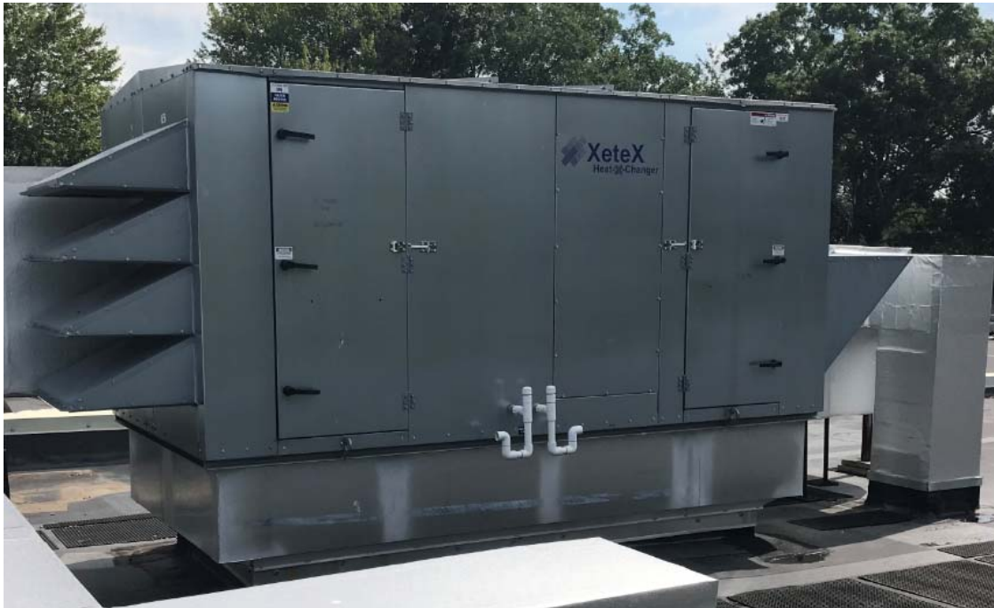
Figure 7- Xetex Energy Recovery Unit
