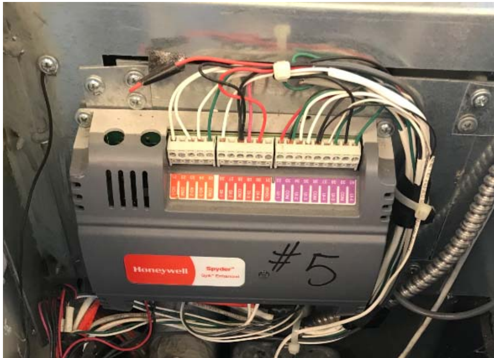
Figure 4- Typical Honeywell controller for UV
