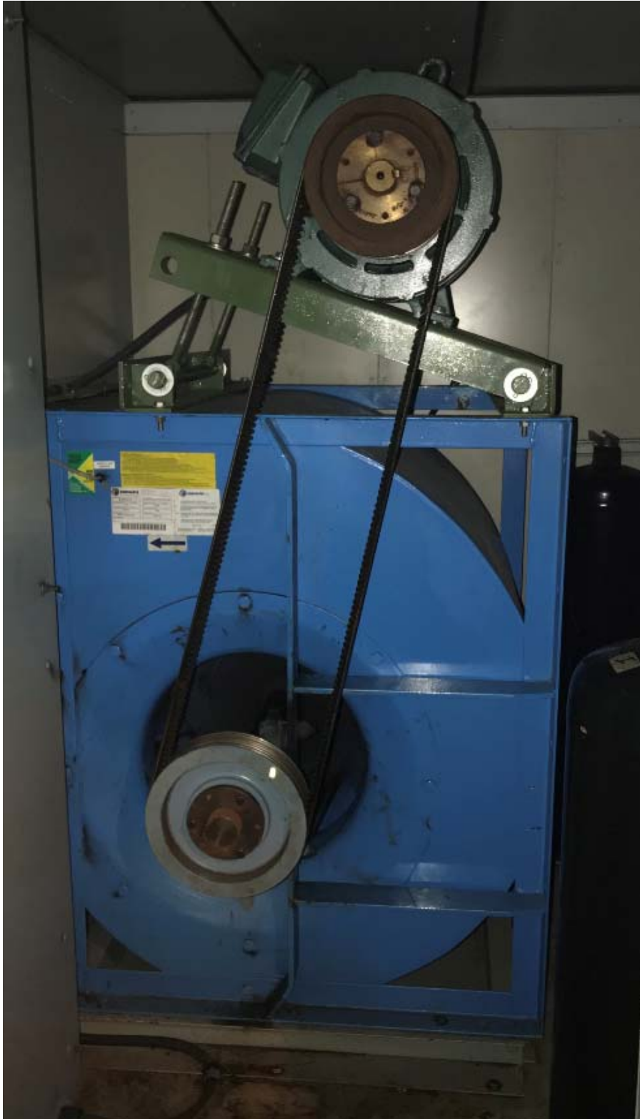
Figure 12-Dectron Unit-Supply Fan section
