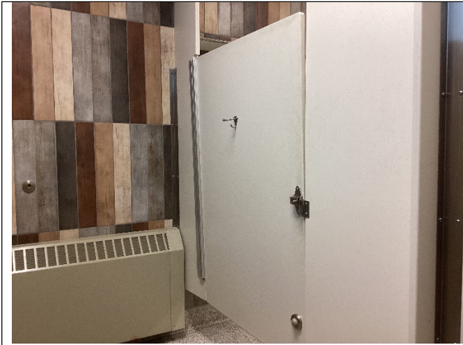
Damaged restroom partition
