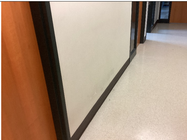
Scuffs on painted surfaces
