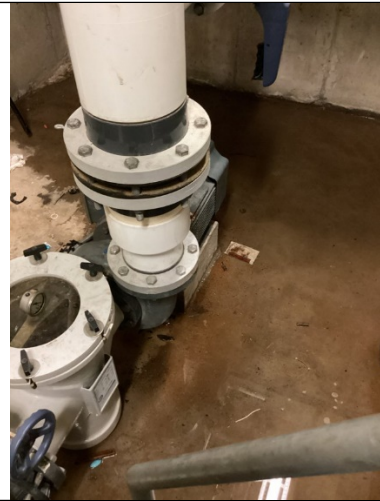
Leaking main pool pump
