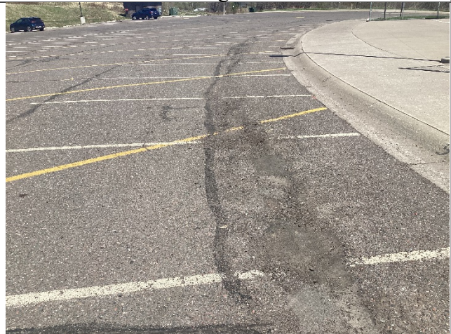
Needed pavement repairs
