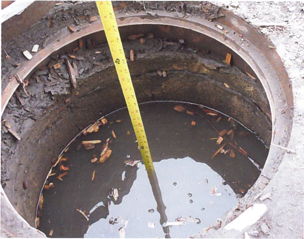
Clogged upstream structure (above)
