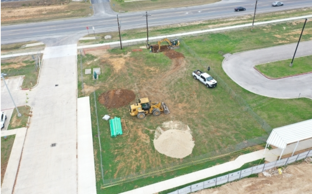
Utilities at Primary
