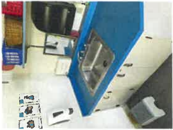
CASEWORK ADJACENT TO TOILET ROOM TO BE MODIFIED IF TOILET ROOM IS EXPANDED TO BE ADA COMPLIANT
