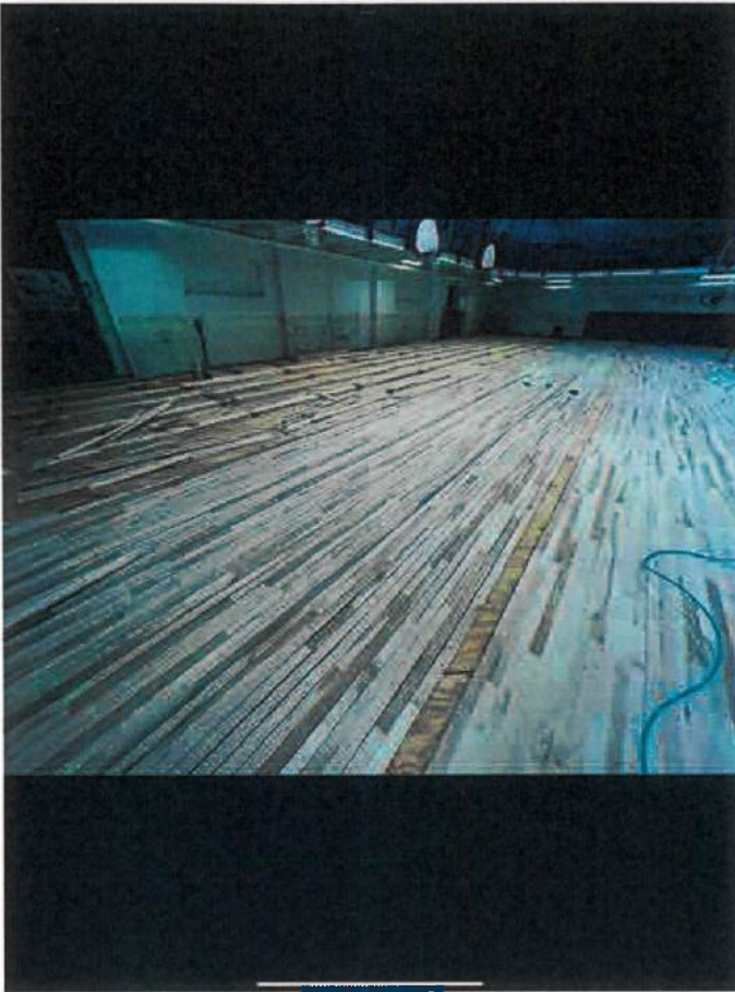
Installation of planks over sheathing Taken on Jan 28, 2025, 3:01 PM CST Added on Jan 28, 2025, 3:02 PM CST Added by Luca Muench
