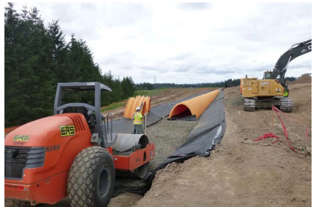
Storm water system - looking west
