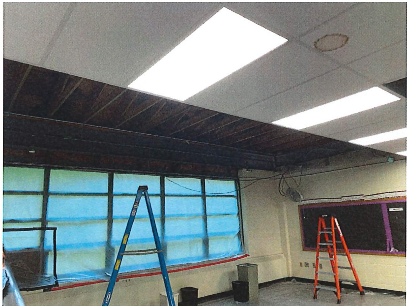
Snow School roof damages ^
