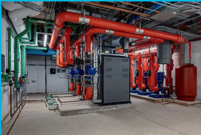
Central Utility Plant Boiler Room
