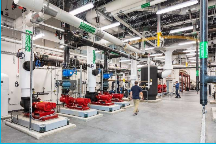
Central Utility Plant
