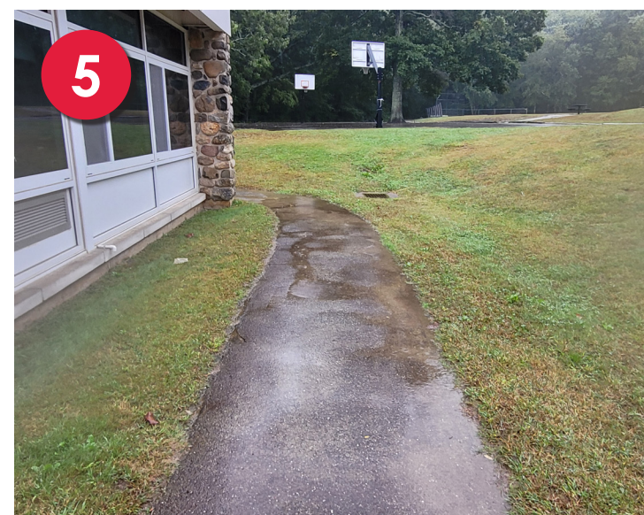
Biofiltration Swale Drainage Area 1
