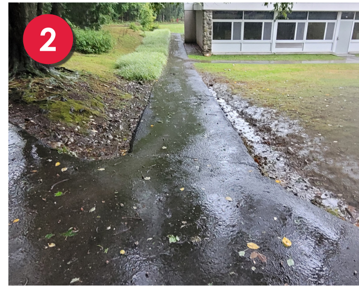
Biofiltration Swale Drainage Area 1
