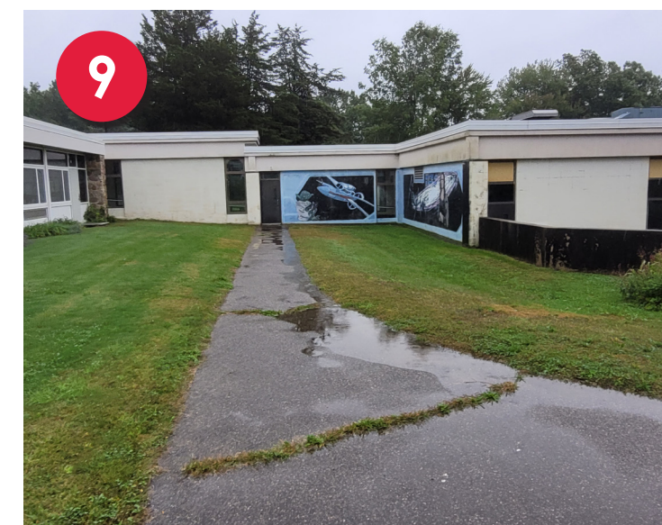
Rain Garden Drainage Area 1
