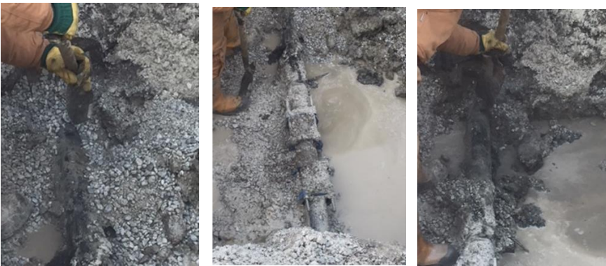
Pictures of 2 nd leak found 12/27/17
