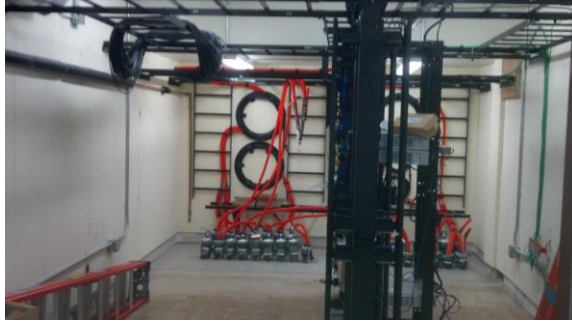
New MDF in "F" Building
