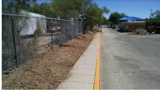
Erosion along east property line
