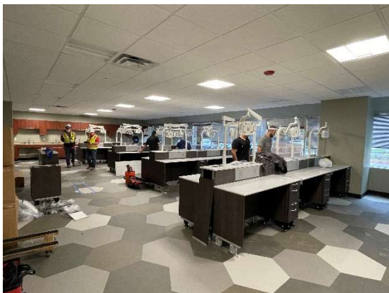
Material Lab Workstations
