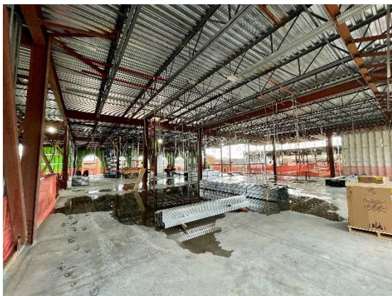
Northend Side of Vet Lounge and Outreach Office Area on 2 nd Floor
