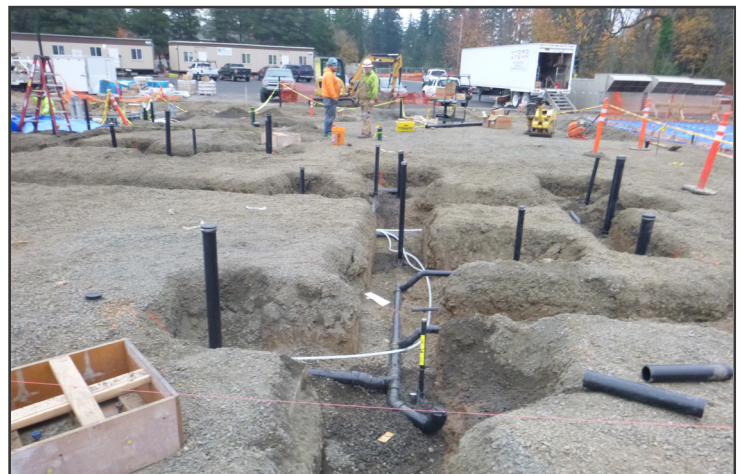
Underground plumbing in kitchen
