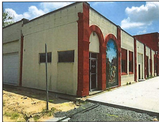
The current Jefferson County coroner's office, at the corner of Barraque and South Main streets in Pine Bluff, has fallen into disrepair and is one of three offices now scheduled for replacement through a public-private partnership authorized by the Quorum Court this month. (Arkansas Democrat-Gazette/Dale Ellis)
