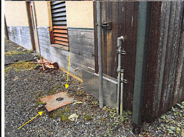
HCSHMG Underground fuel tank access. Equipped with Veeder-Root monitoring system. System appeared to be functioning properly.
