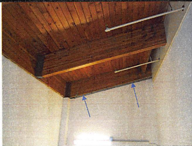
HCSHMG Signs of water intrusion on wood glulam beam. Need to determine source. Is this a recent event?
