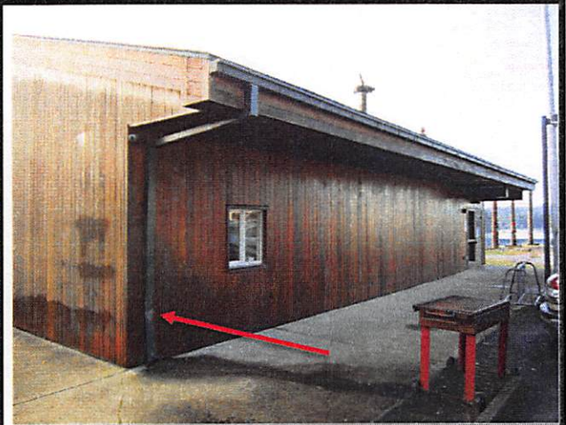
HCSES Partly crushed rain gutter. Underground drain appears to be out of order.
