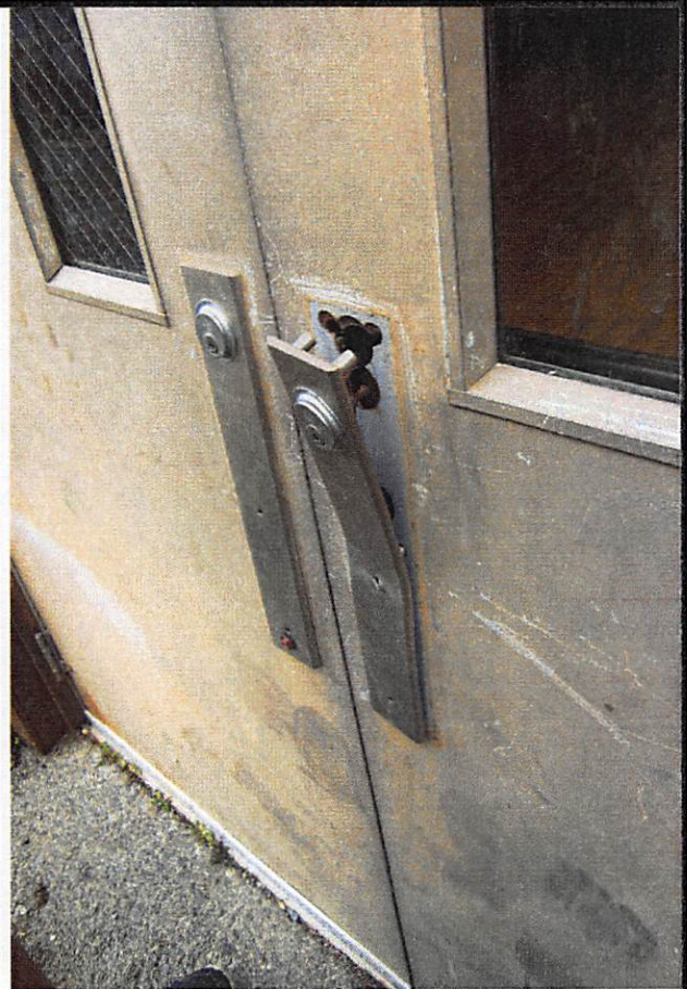
HCSHMG Act of vandalism. Immediate access to gym area. Needs repaired.
