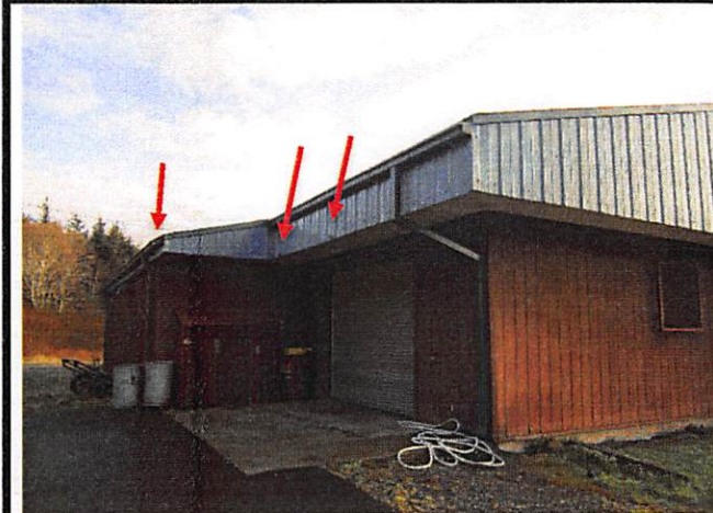
HCSJSHS Surface damage to facility.
