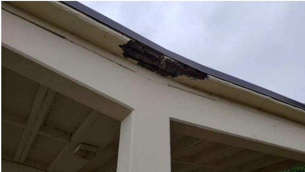
Figure 5: Deteriorated concrete at front entry canopy
