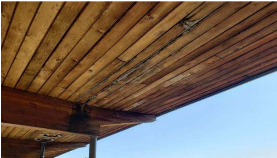
Figure 2: Damage at covered walkway areas
