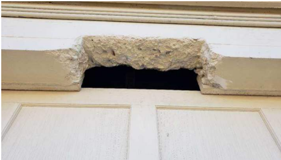
Figure 6: Damage to concrete headers
