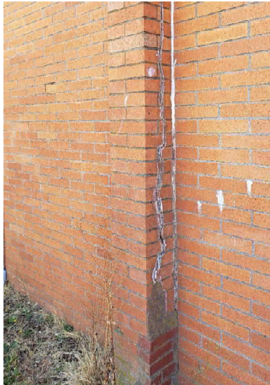
Figure 3: Damaged brick veneer
