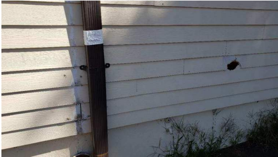
Figure 1: Damage to siding and downspout
