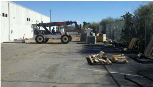
HVAC Unit Placement
