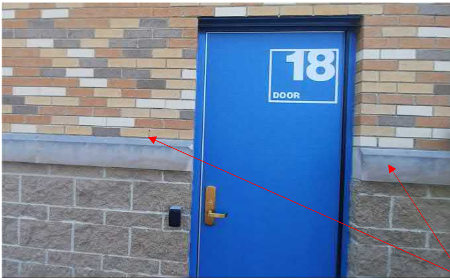
Figure 14: General Areas of cracked mortar in need of repair. Tuckpoint and seal open joints. Clean Sills.
