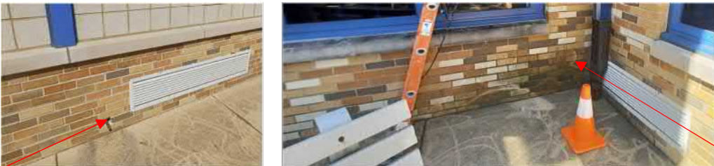
Figure 26: Areas requiring brick replacement, tuckpointing and cleaning. Existing, drying and cracking sealant at sills in need of re-sealing with new elastomeric sealant.
