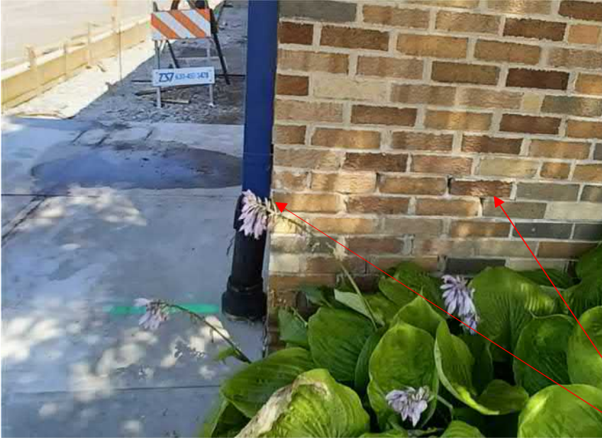
Figure 32: General areas of cracked, broken brick in need of replacing and tuckpointing.
