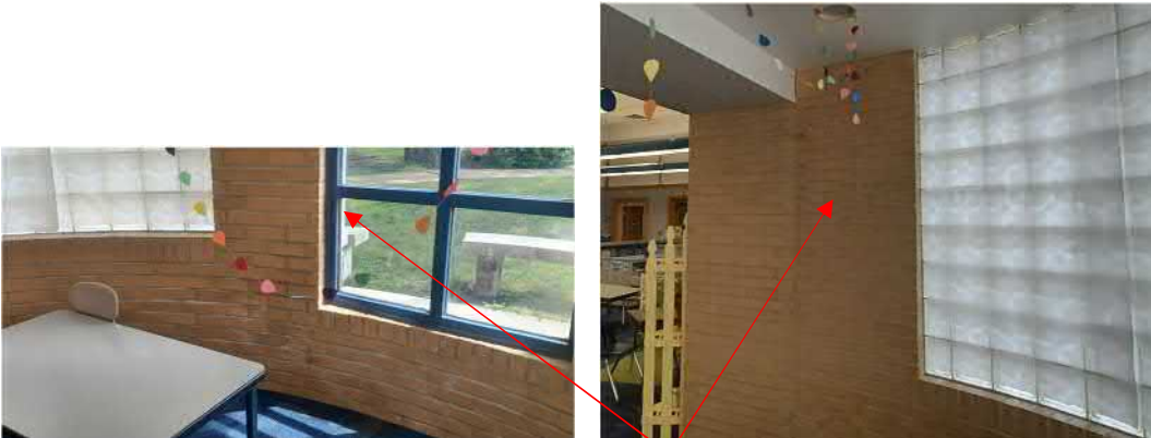
Figure 21: Evidence of water infiltration / efflorescence.
