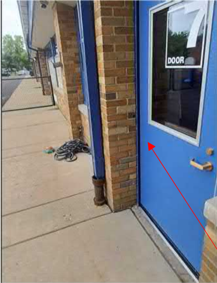
Figure 29: Area of mortar in need of tuckpointing.
