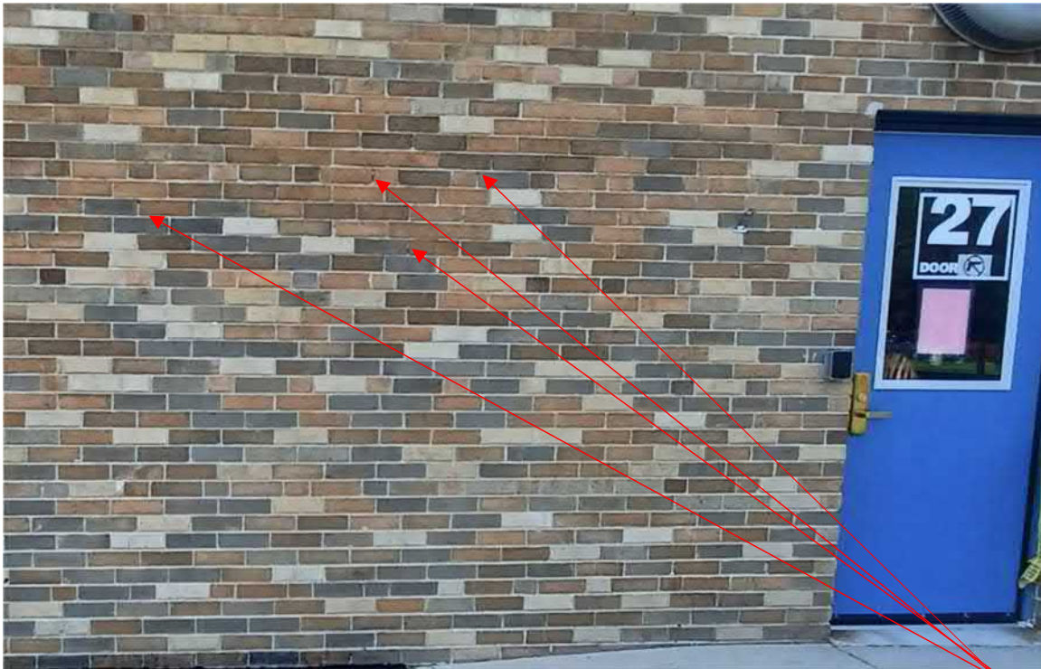
Figure 4: General Areas of cracked mortar in need of repair and tuckpointing of broken and open joints.
