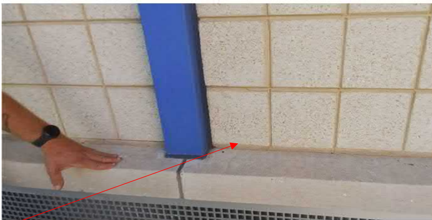
Figure 31: The cast stone sills appear to be 'drooping' at the center of the larger unit ventilator grilles, which is cracking the mortar between the wall and Smooth face CMU window infill. The 1955 and 1993 details show steel lintels for the smaller grilles, but none were found for the larger grilles. Further investigation is required.
