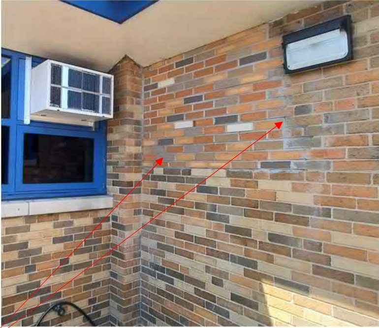
Figure 5: Previously tuckpointed area that could be improved, re-pointed to match existing joints.
