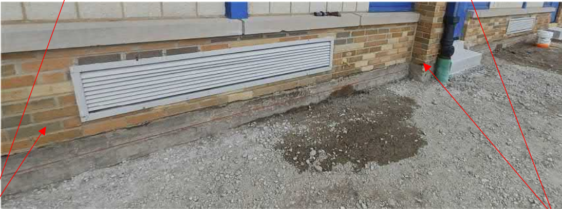
Figure 36: Bottom 2 or 3 courses of brick in need of tuckpointing. Typical this area of North elevation.
