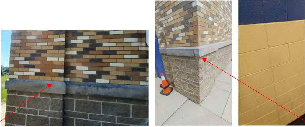
Figure 13: Vertical control/expansion joints at 1993 construction gymnasium, to be removed and re-sealed with new sealant, outside and inside. Cast stone sills are in need of repair and cleaning. Joints in need of being ground out re-pointed and re-sealed.
