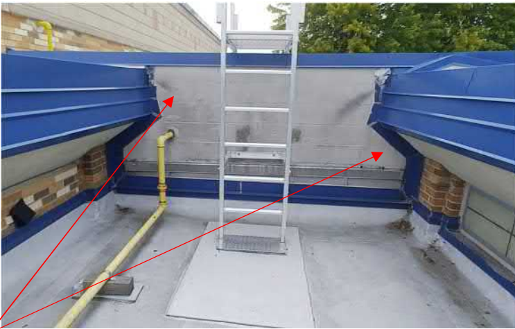
Figure 49: CMU in need of repair, tuckpointing and painting.
