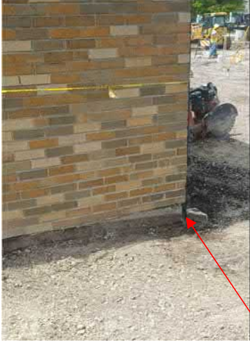
Figure 1: Area of damaged foundation and cracked mortar joints @ Southwest corner in need of repair and tuckpointing.
