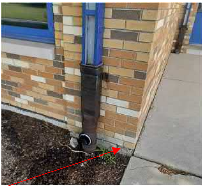
Figure 16: Foundation wall in need of repair.
