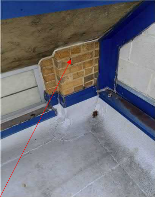
Figure 46: Various brick 'piers' with areas of broken and open mortar joints in need of repair and tuckpointing.
