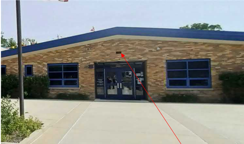
Figure 37: New bricks needed to replace missing bricks above door #2.
