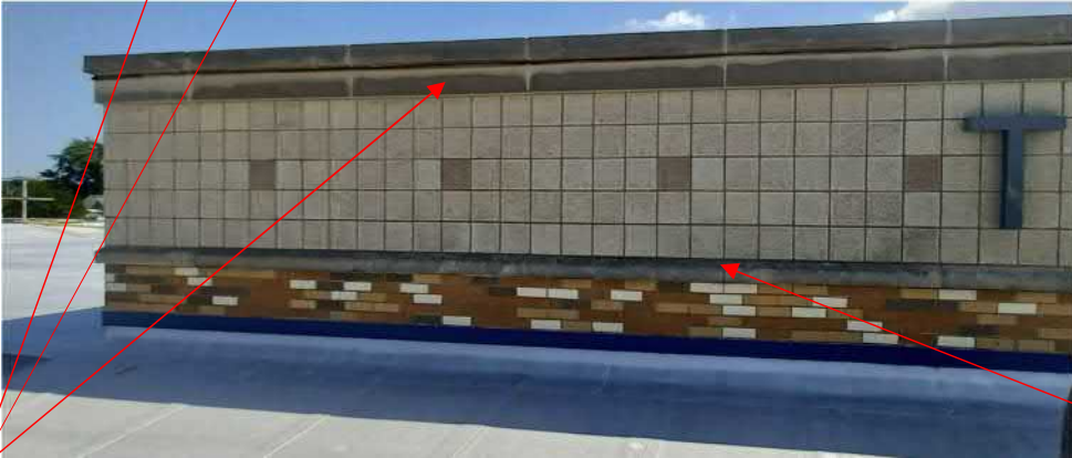
Figure 43: Stone sills and smooth face CMU in need of power washing. Stone sills joints in need of joints being ground out and re-sealed with elastomeric sealant.
