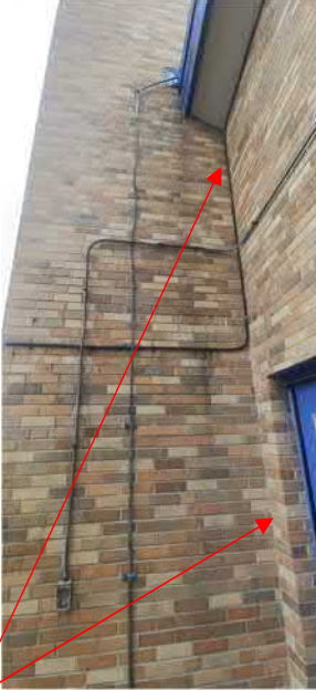
Figure 7: General area in need of tuckpointing and a few broken / cracked bricks..
