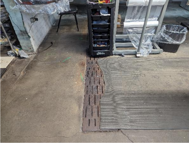
View of the floor drain in the central portion of the main building.
