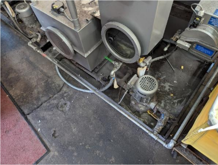
View of dark stained concrete near a drycleaning machine in the southwest corner of the main building.
