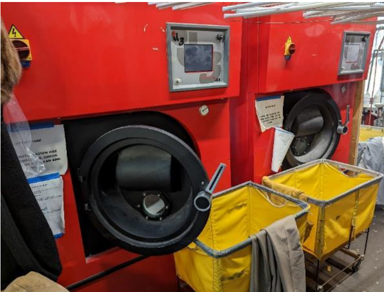
View of the drycleaning machines in the southwest corner of the main building.
