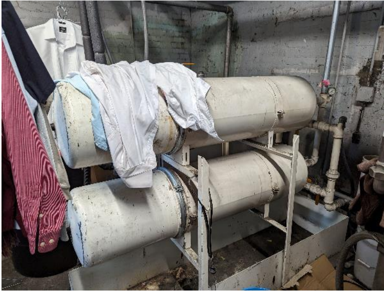
View of the filtration vessels and secondary containment in the southwest corner of the main building.
