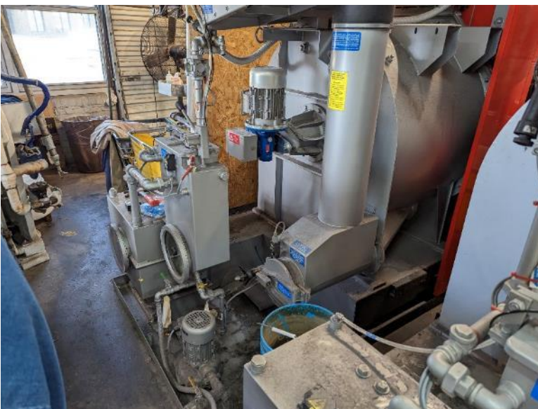
View of the back of the drycleaning machines in the southwest corner of the main building.
