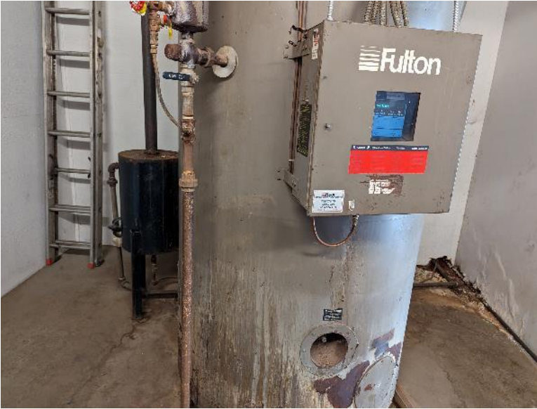
View of the active boiler in the northwest corner of the storage building.
