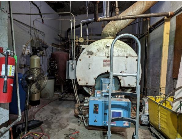
View of the abandoned boiler in the northern portion of the main building.
