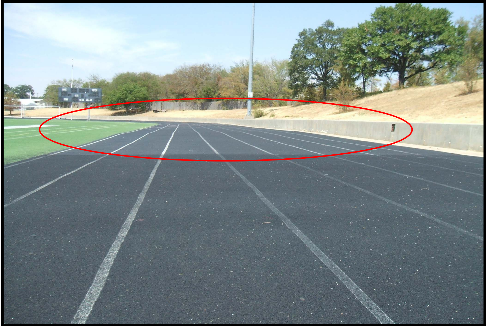
Uneven surface on track and field
