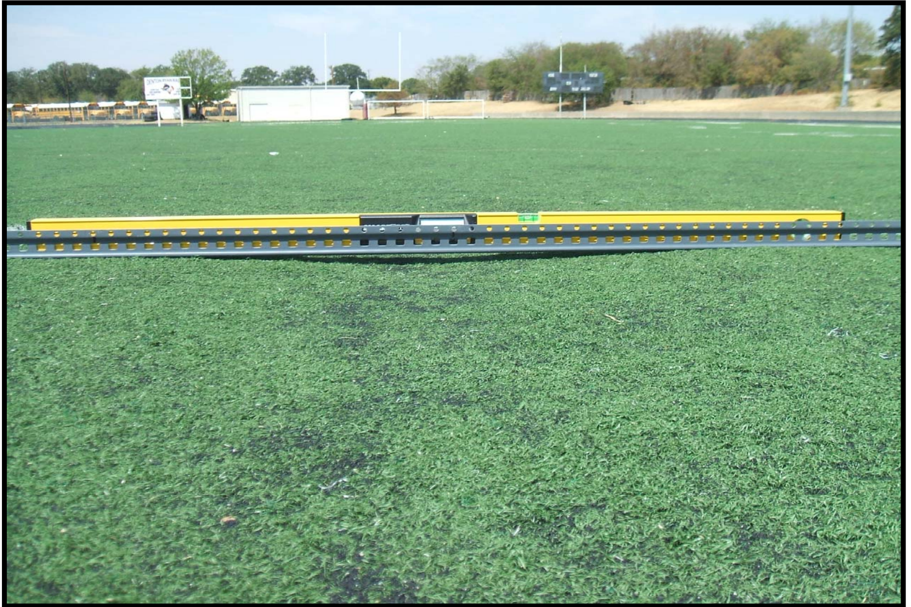
Movement in subgrade
