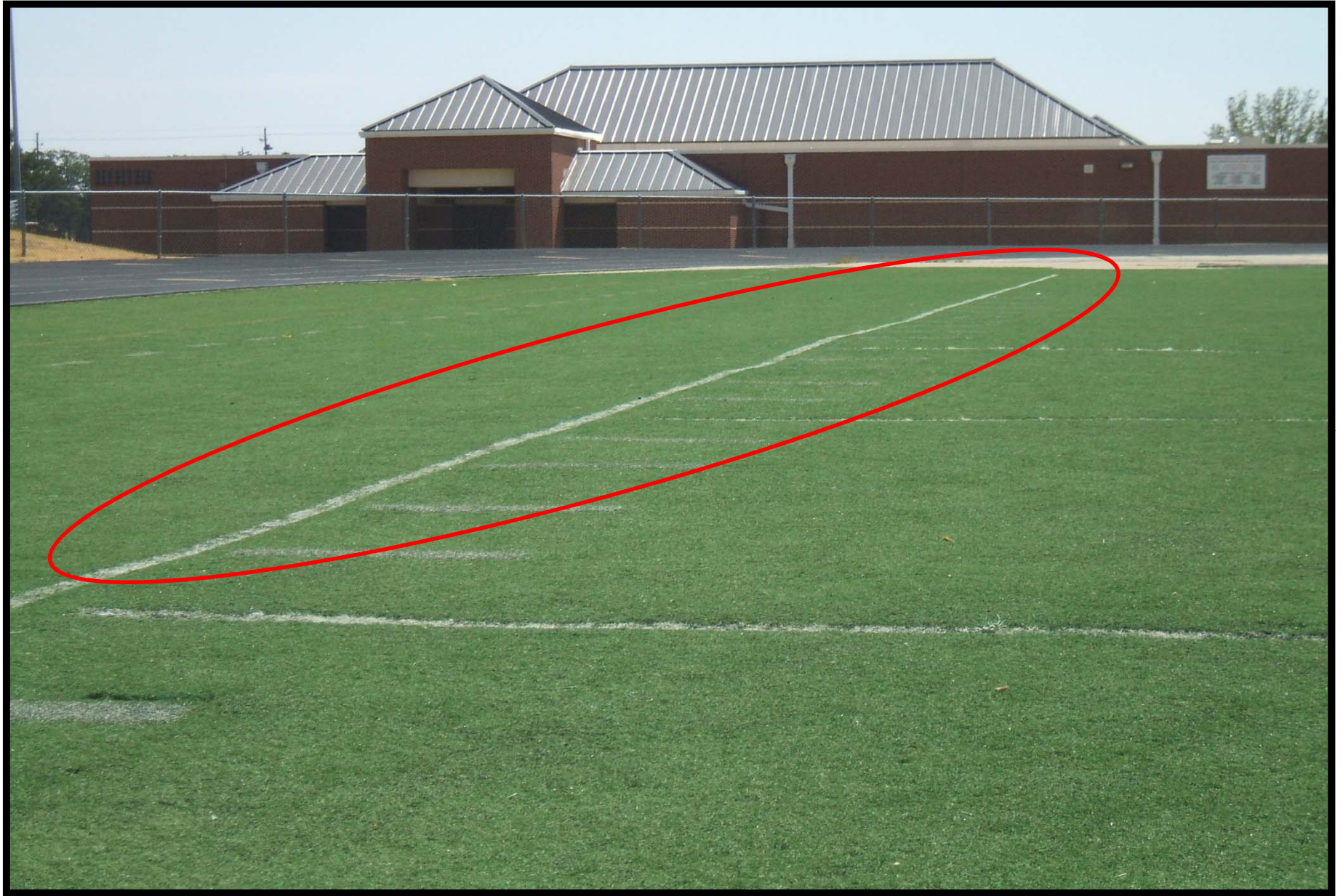
Uneven playing surface
