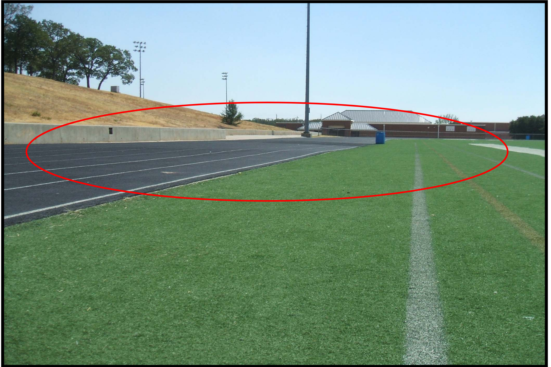
East side of track and field has experienced movement
