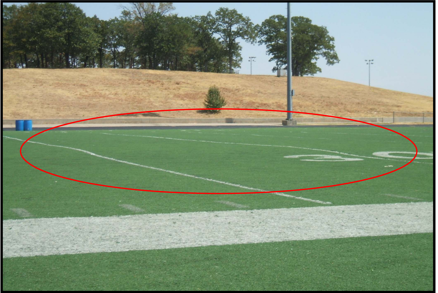
Subgrade movement resulting in uneven playing surface
