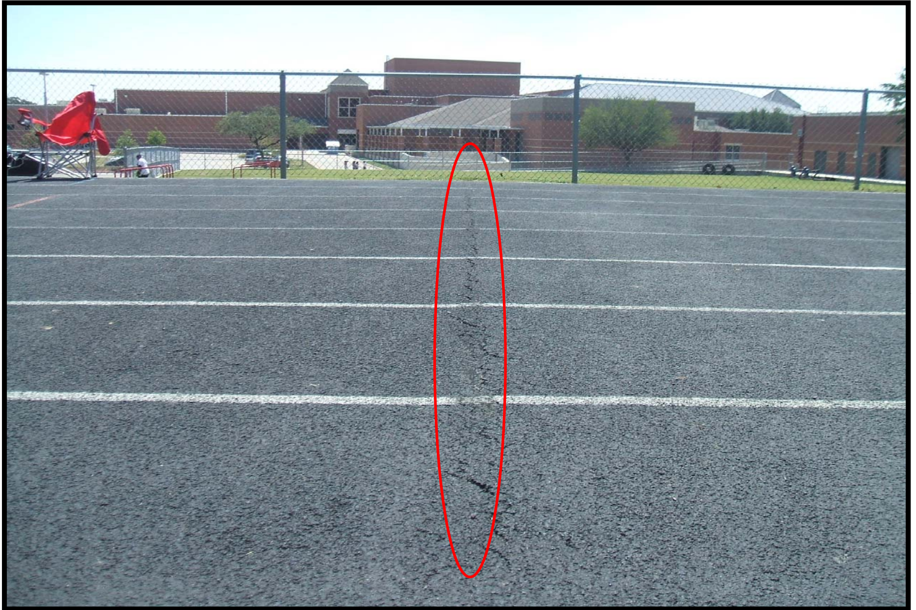
Movement in base resulting in surface pushing upward
