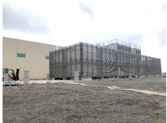
Cooling Towers at CUP
