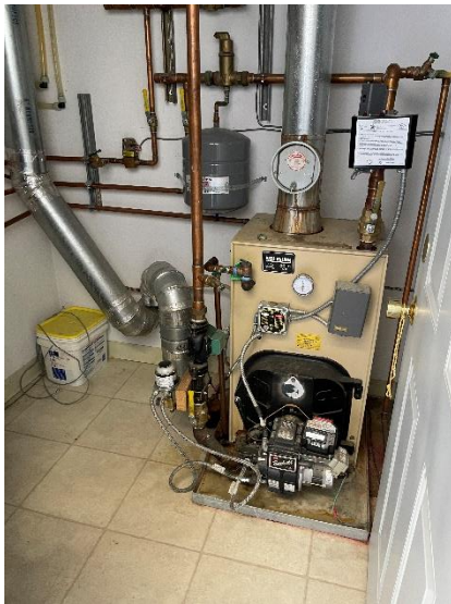
Photo M18 – Boiler
