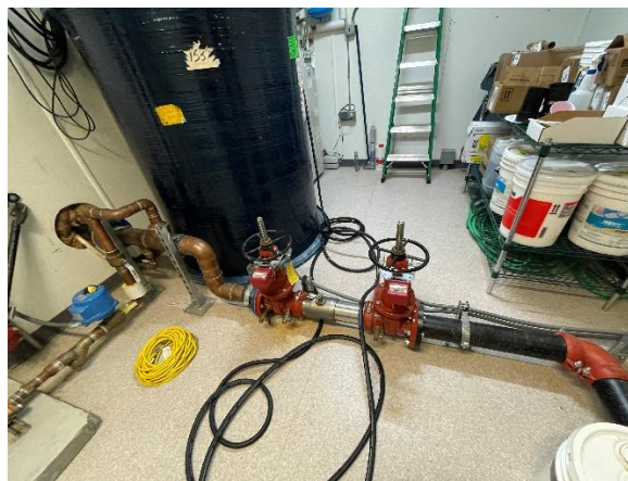
Photo M14 – Water Service
