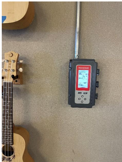
Photo M11 – AHU Temperature Controller
