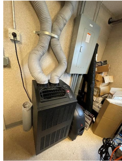
Photo M10 – IT Room AC
