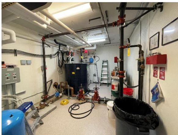
Photo M13 – Sprinkler Riser
