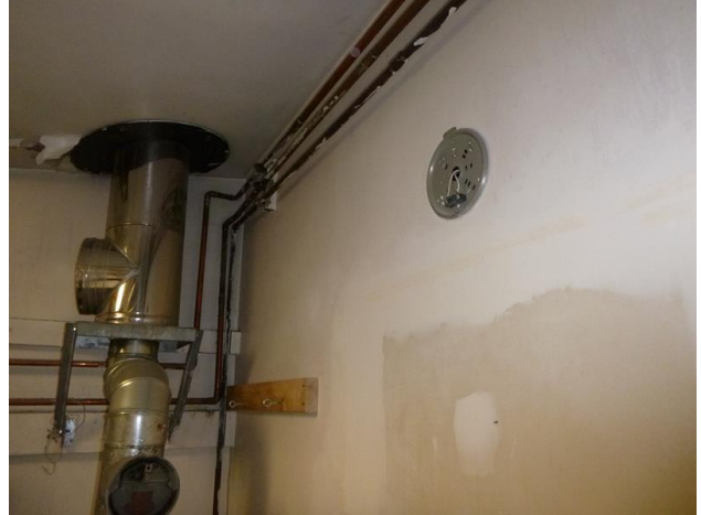
Photo E6 – Typical Missing Smoke Detector
