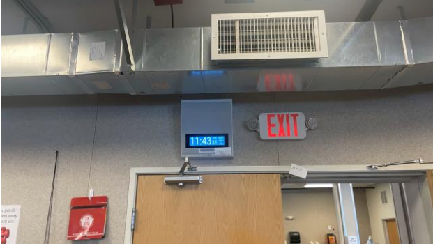
Photo E6 – Intercom Speakers and Wireless Clocks
