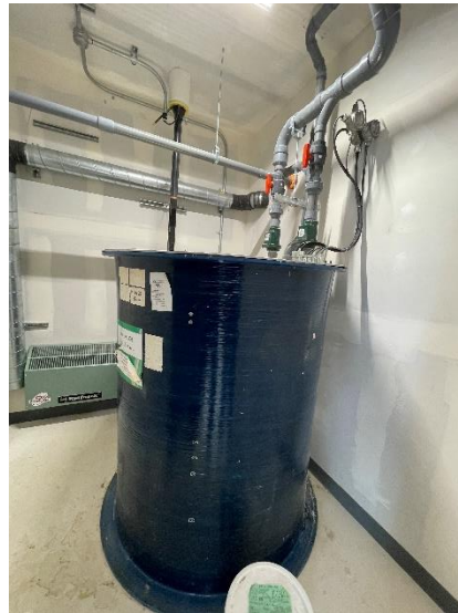
Photo M2 – Area Lift Station
