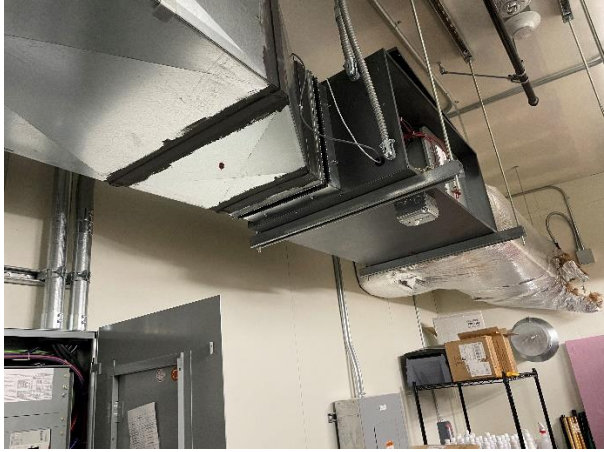
Photo M5 – AHU w/Electric Coil
