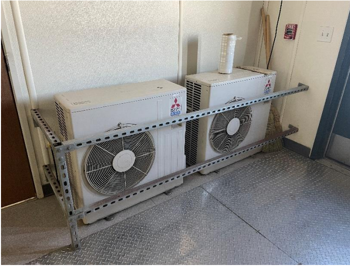
Photo M9 – Electrical Room Condensing Units
