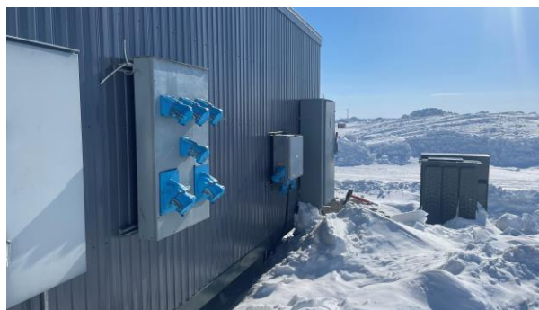
Photo E4 – Exterior service and standby connections
