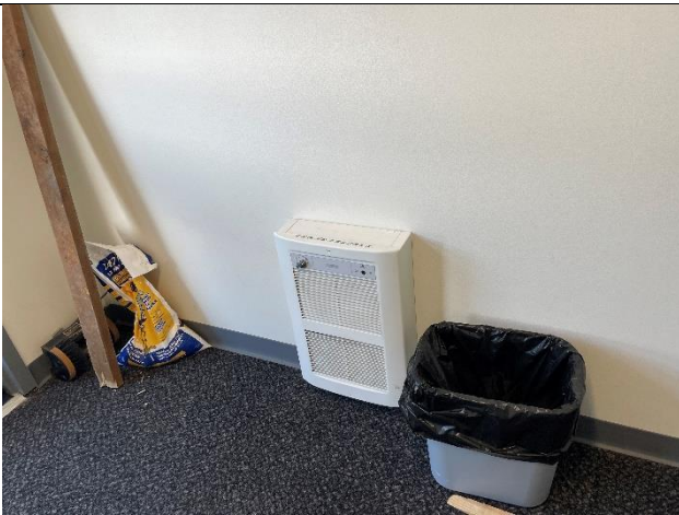
Photo M7 – Electric Wall Heater
