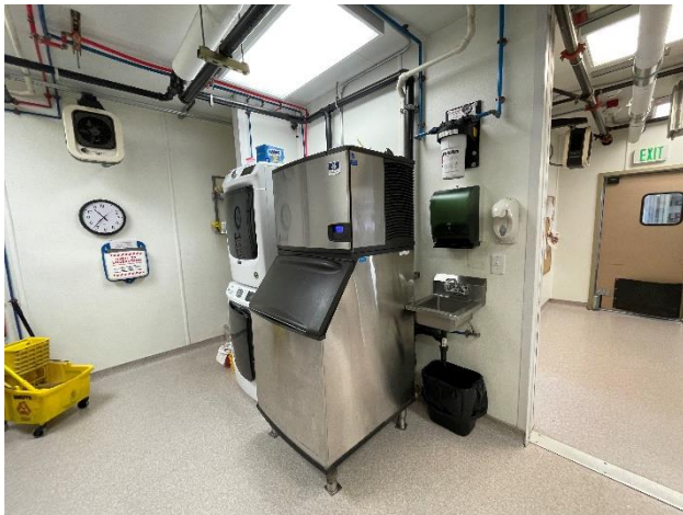
Photo M3 – Icemaker and Lift station
