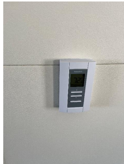
Photo M12 – Typical Thermostat
