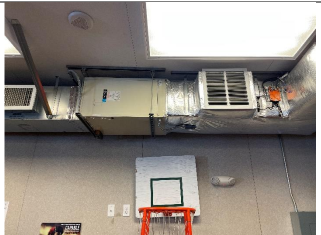
Photo M8 – AHU in Recreation Area
