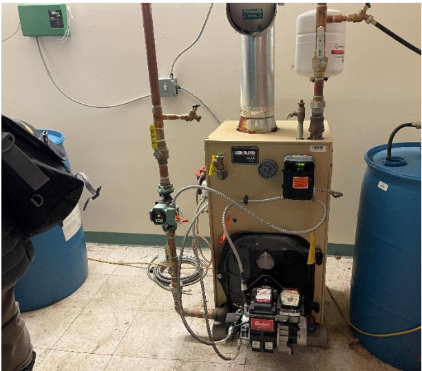
Photo M15 – Old School Boiler
