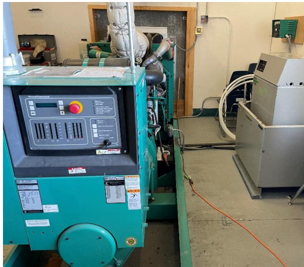
Photo M16– Old School Generator / Day Tank
