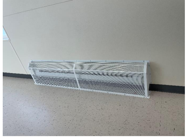
Photo M6 – Corridor Electric Baseboard
