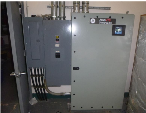
Photo E1 – Electrical Service Disconnect and ATS
