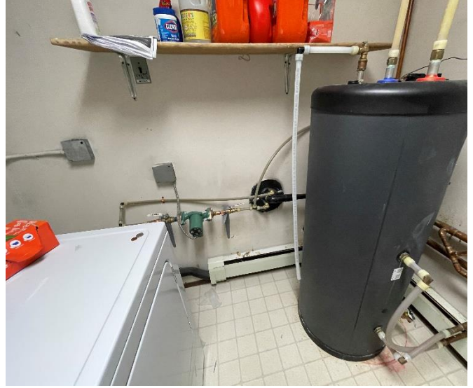
Photo M16– Hot Water Generator
