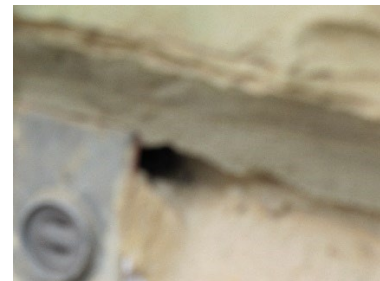
SMALL HOLE IN WALL NORTH SIDE
