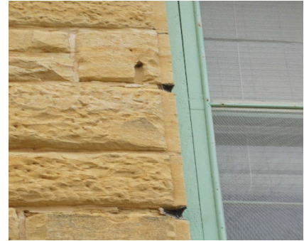
SMALL HOLES NORTH SIDE
