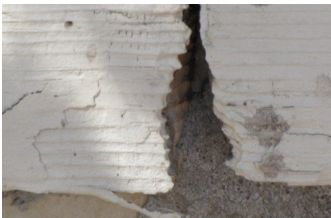
west side, lower left cracking.
