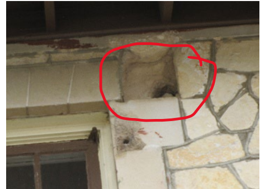
ROCK MISSING BY SECOND FLOOR WINDOW
