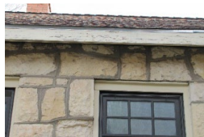
fascia needs painting
