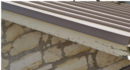
So. side fascia needs painting
