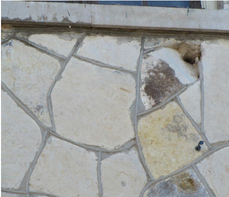
HOLE UNDER 2 ND STORY WINDOW
