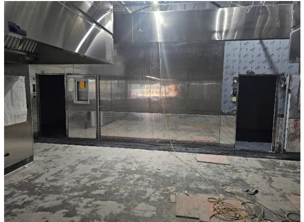
Kitchen Walk In Coolers
