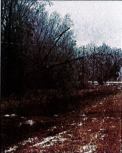
that traveled from near and far, 27,750 feet of power lines. SWEC reported that due to Storm, page 7
