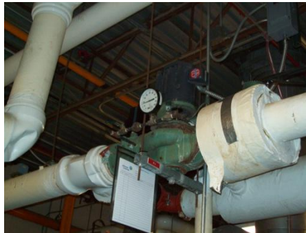
Primary Boiler Pump
