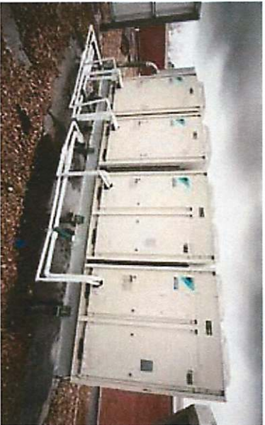
HVAC Units in Need of Replacement
